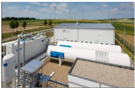
Power to hydrogen- PEM Electrolyser
